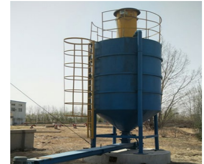
Inner Mongolia Consun East Desulphurization and Dust Removal System
